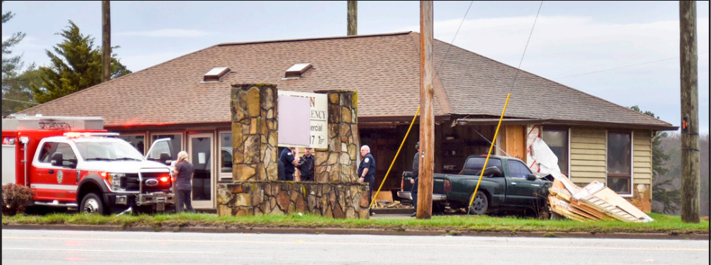
A Toyota Tacoma knocked out the front and side walls of a corner office in the former HQ for Robert F. Jackson Insurance Agency the morning of March 2. Photo by Todd Forrest
